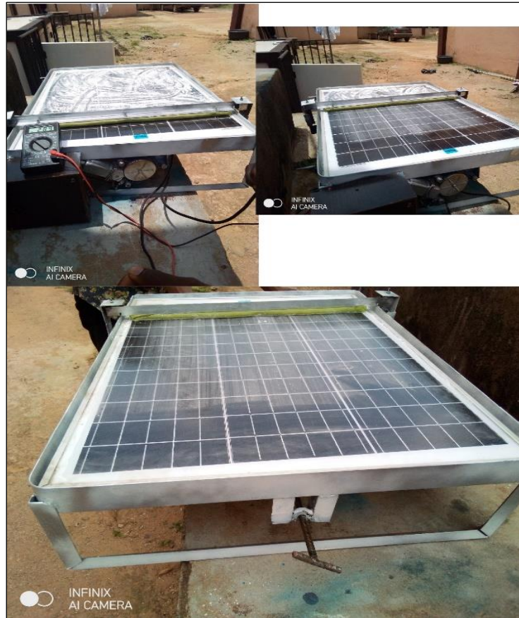
Figure 2: Automated Solar Panel Cleaning System in operation
